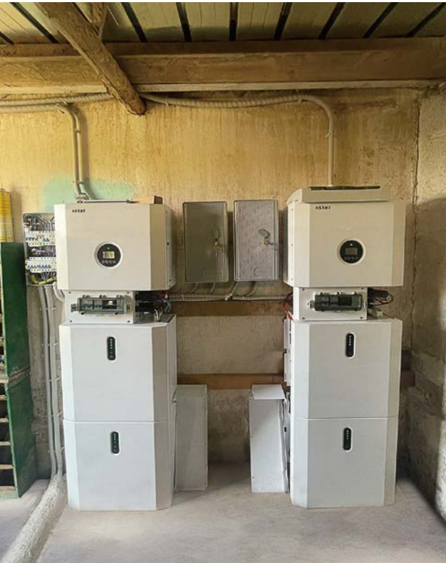
05 Residential ESS Project in Italy
