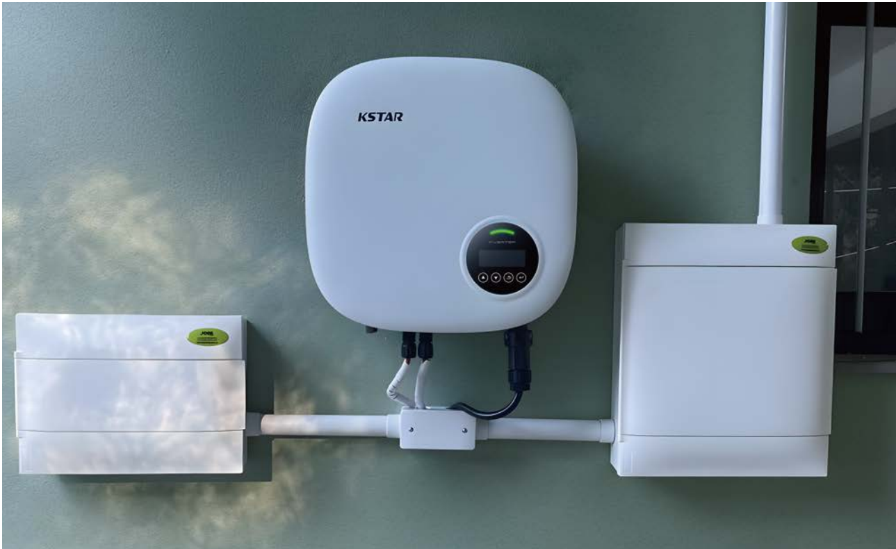
07 Residential Solar Project in Brazil
