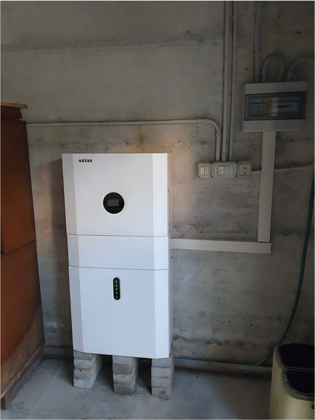
01 Residential ESS Project in Italy
