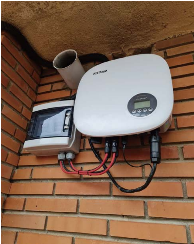
04 Residential Solar Project in Brazil
