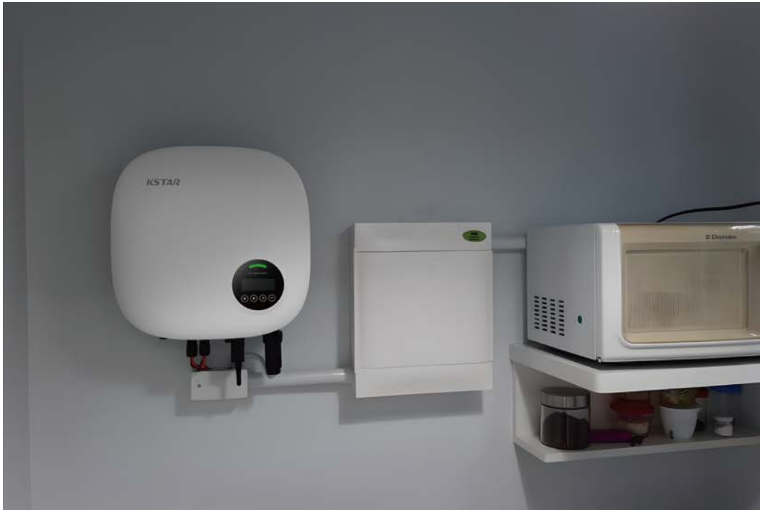
10 Residential Solar Project in Brazil
