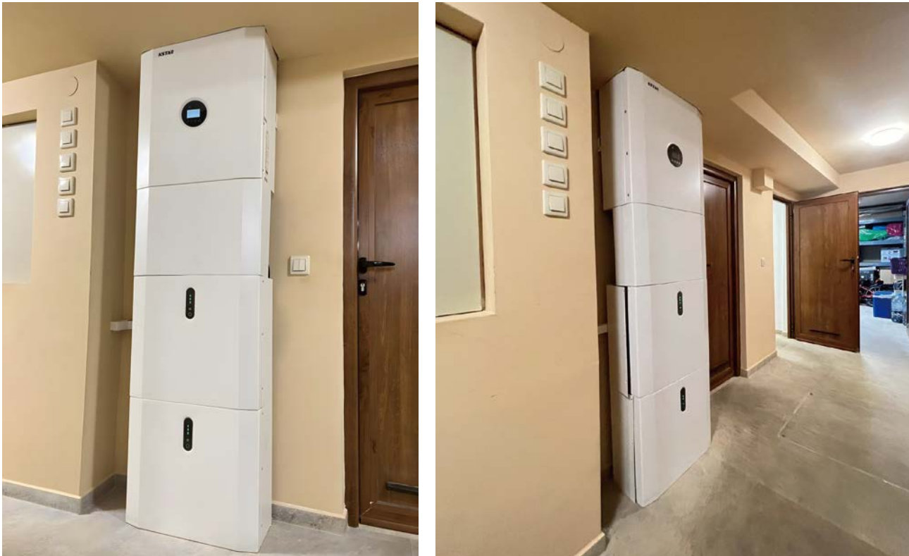
03 Residential ESS Project in Bulgaria
