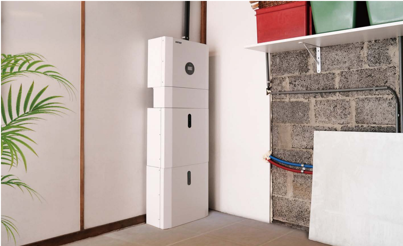
06 Residential ESS Project in the Netherlands
