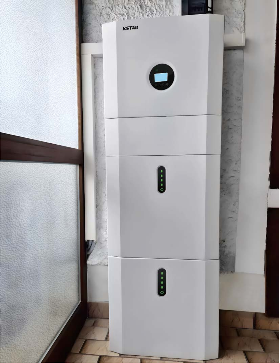
02 Residential ESS Project in Italy
